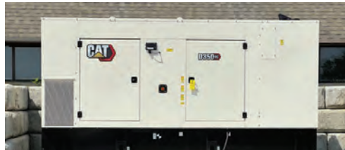
The rebuilding of the electrical room meant replacing the damaged main breaker and other electrical equipment and installing a new generator (pictured).
