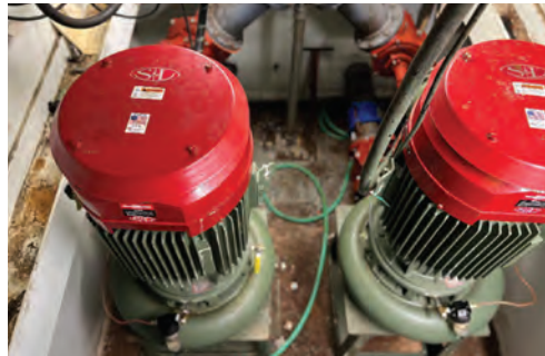
The newly installed pumps at pump station 4.
